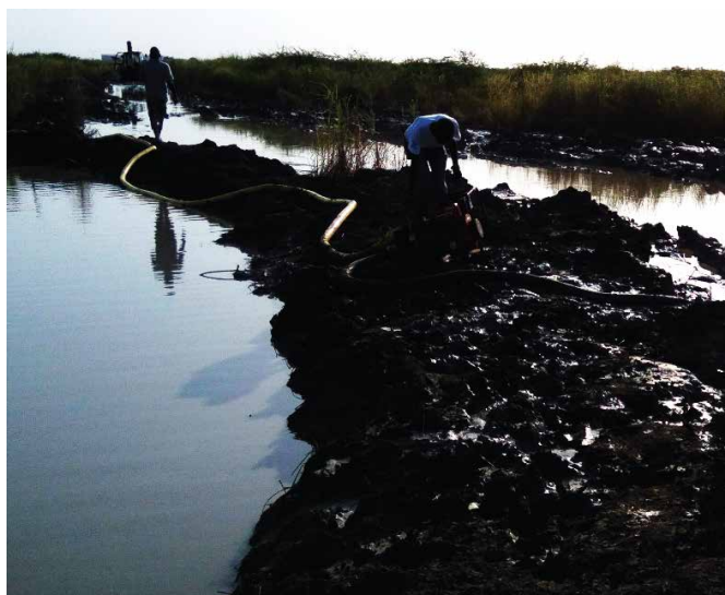
Setting out and pumping water from the road towards Liquid waste water stabilization pond outside base before rehabilitation. IOM/Makhatsa 2017.
